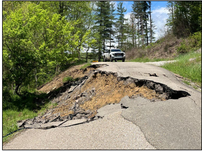
Athens County Road Slip Following Heavy Storms During Spring 2025 (Photo Courtesy of Athens County EMA)
